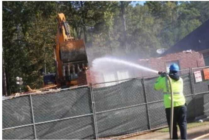
Figure 10. Example of construction site watering and boundary chain link fence with mesh material affixed. 8
