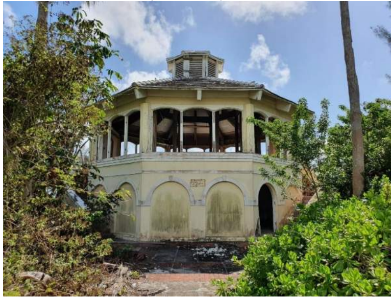
Figure 40(a-d). Sample location Pool Kitchen, ACM samples collected from pipe insulation and drywall, lead samples taken from exterior paint
