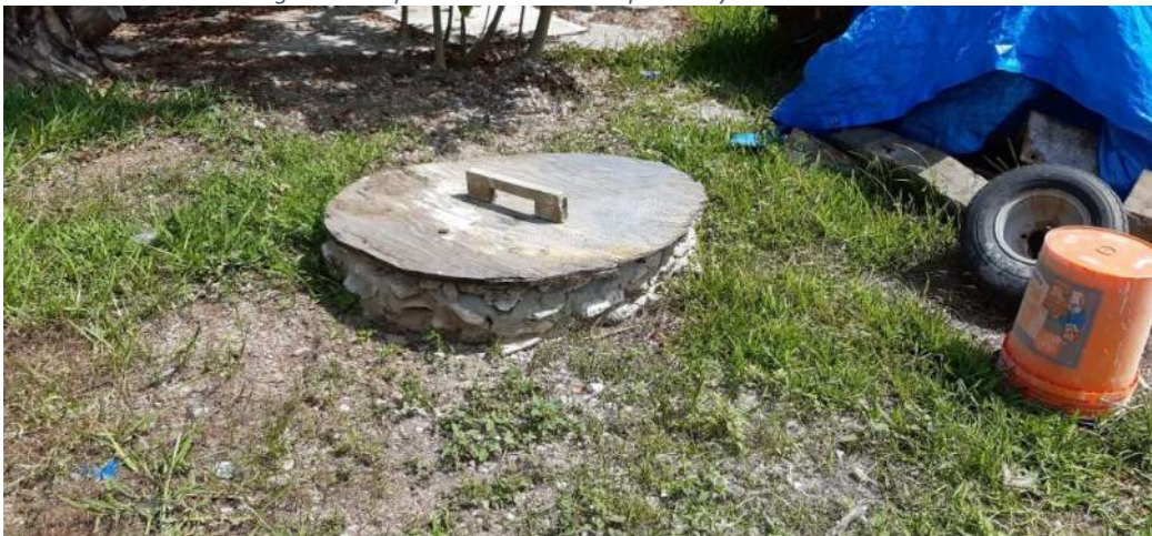
Figure 38. Septic tank within close proximity to marina basin
