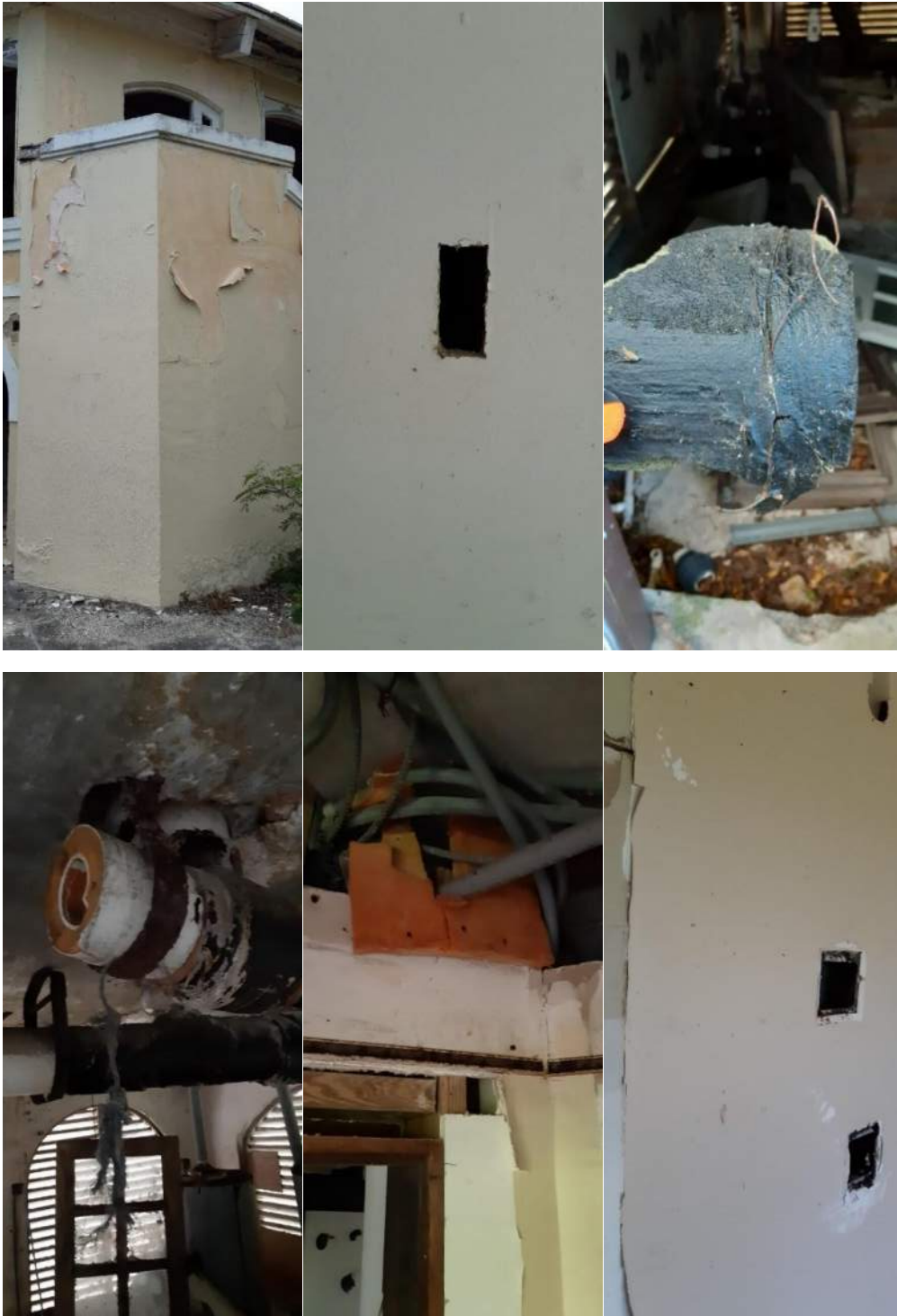
Figure 43 (a-f). Lead sample exterior Pool Kitchen; ACM sample interior Pool Kitchen; ACM sample pipe insulation Pump House; ACM sample pipe insulation Pump House; ACM sample AC insulation Great House 2; ACM and lead sample interior Great House 2.
