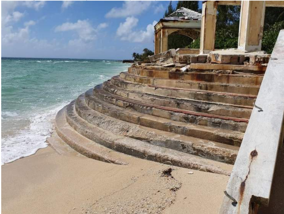
Figure 16. Coastal infrastructure impacted by coastal erosion and sedimentation
